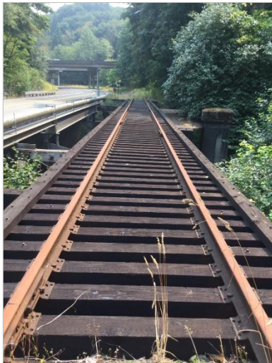
Photo 46. Rail bridge over BNSF Railroad with I-5 overpass in the background, looking east.
