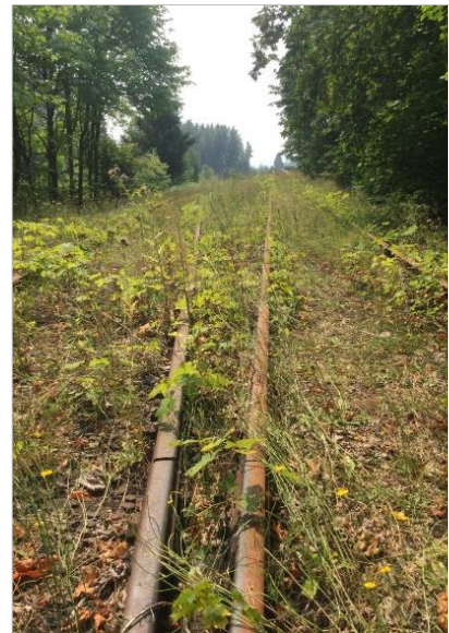
Photo 40. View of double track north of trestle with slight vegetation growth, looking south.
