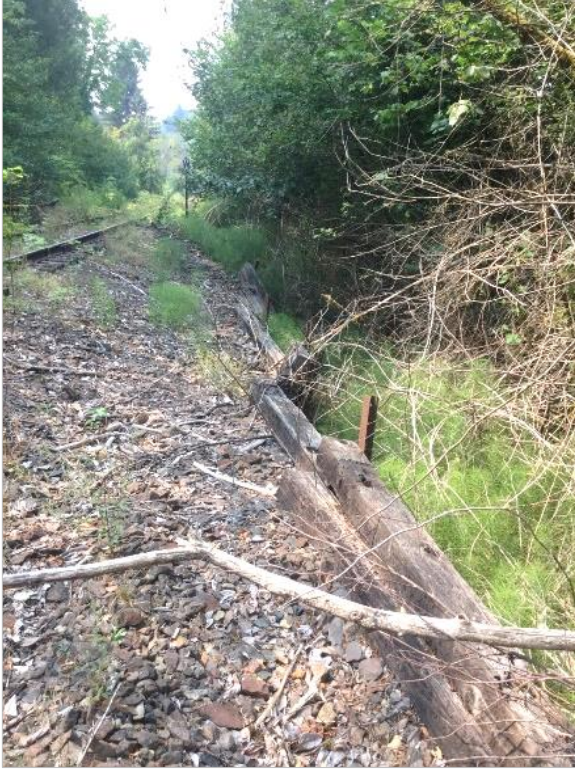
Photo 50. West side of rail berm with rail tie retaining wall, looking south.
