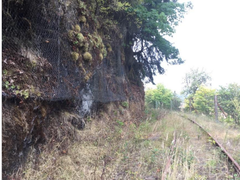
Photo 45. Corridor on north side of Rocky Butte with mesh rock protection, looking west.
