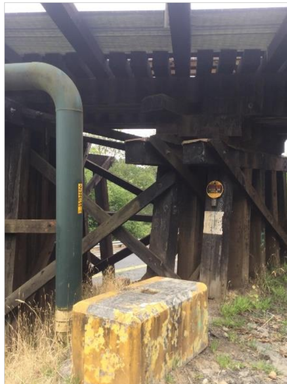
Photo 36. Natural gas pipeline on north side of the trestle, looking south
