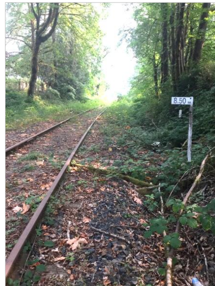
Photo 63. Milepost 8.5 at the northern terminus of the Patriot Woods Rail corridor, looking north.
