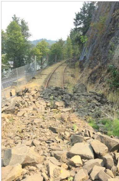
Photo 42. Rockfalls on track along Rocky Butte, looking north.
