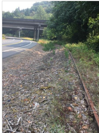
Photo 47. Vegetation growth over rail with I-5 overpass in background, looking east.
