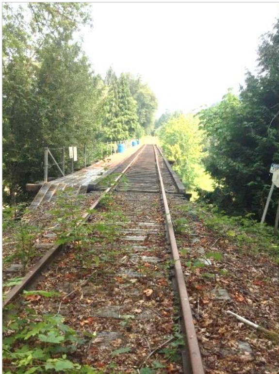
Photo 52. Top of trestle over an unnamed creek and Evergreen Road, looking north.
