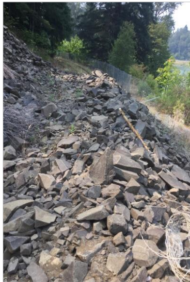
Photo 43. Southern rockfall on track along Rocky Butte, looking south.
