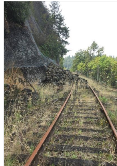
Photo 44. Northern rockfall on track along Rocky Butte, looking south.
