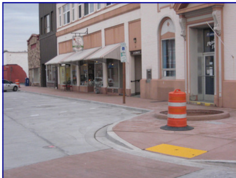
City of Castle Rock is completing a multi-phase infrastructure project throughout its downtown
